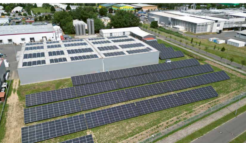
Photovoltaic plants on roof and open areas, Elsterwerda plant
